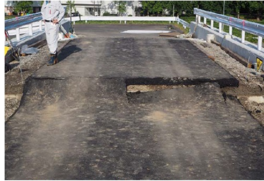
Fig.5 The step after experiment (There are reinforcing materials on the left side.)
