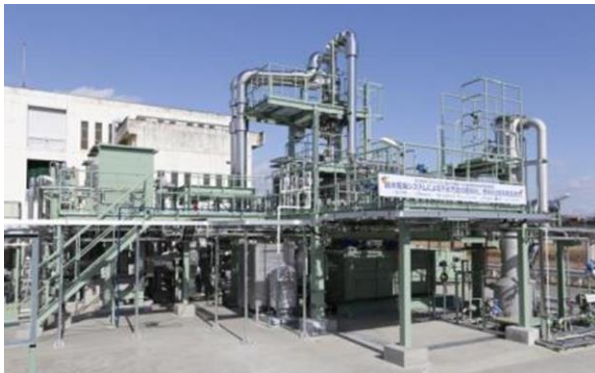
Figure 3 Appearance of full-scale demonstration plant (Dehydration and Drying Technology)
