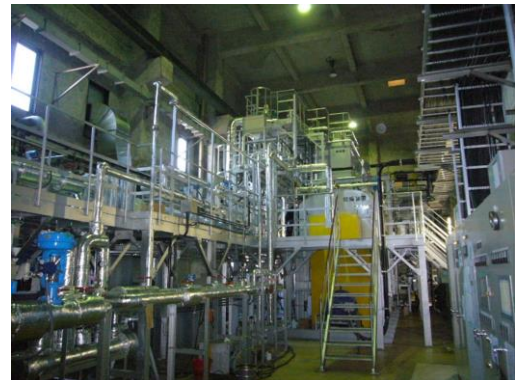
Figure 4 Appearance of full-scale demonstration plant (Self-heat Drier Technology)
